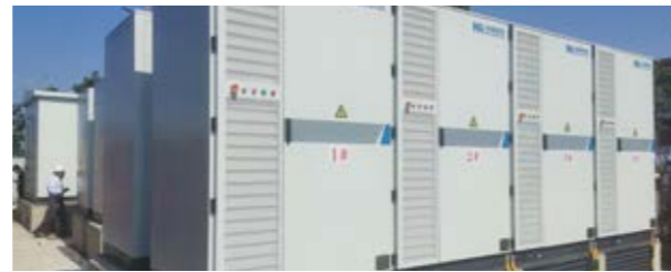
Energy Storage Project
